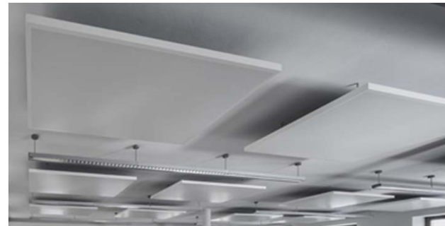
2. Ceiling canopy/panels – Cat B
